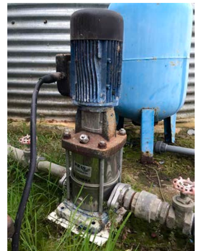
Vintage Vertical Pump with galvanised steel pipework, gate valves and brass NRV. Expansion vessel in the background.
