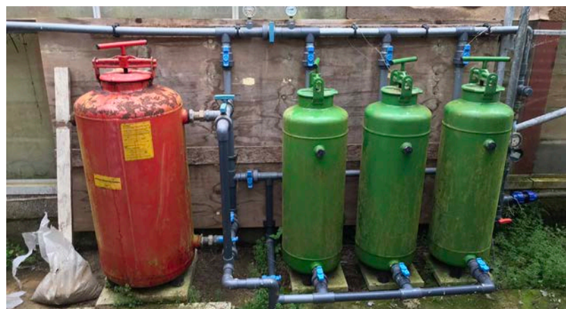
Sand filter installation for stored collected rainwater filtration, green filters are in paralel followed by the red filter which contains sand and ground biochar.
