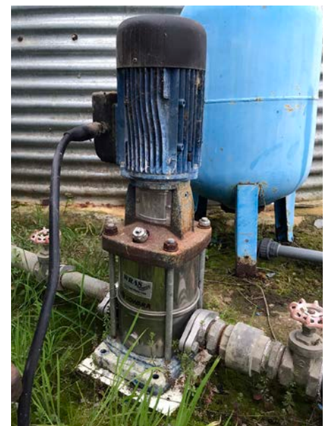
Vintage Vertical Pump with galvanised steel pipework, gate valves and brass NRV. Expansion vessel in the background.
