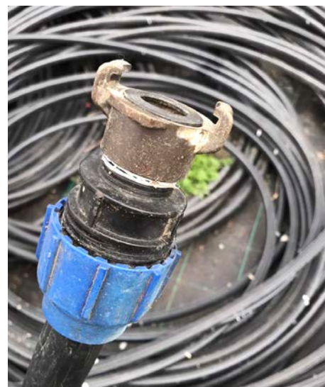
Brass quick connector threaded to poly compression fitting on 32mm LDPE pipe.
