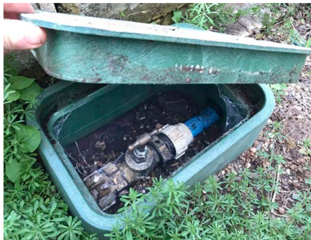
Incoming mains supply stop cock in a ground access box, Hankham Organics
