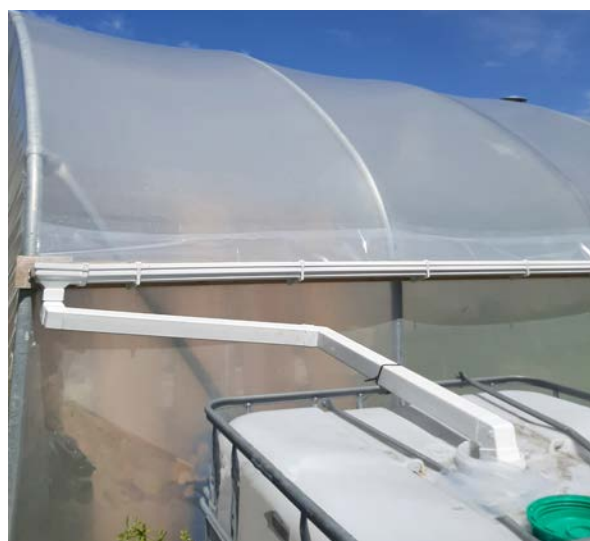
Retro-fitted water harvesting from polytunnel
