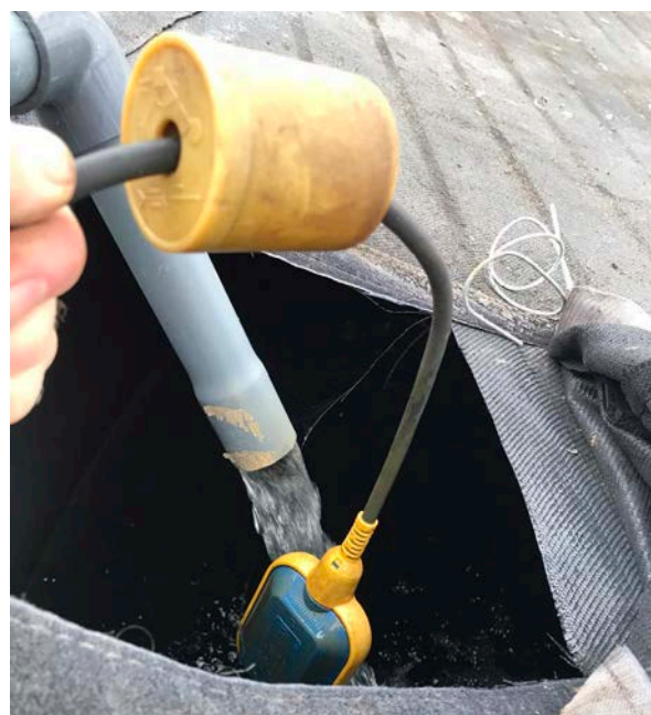
Float switch used to automate tank filling from rainwater storage, Hankham Organics
