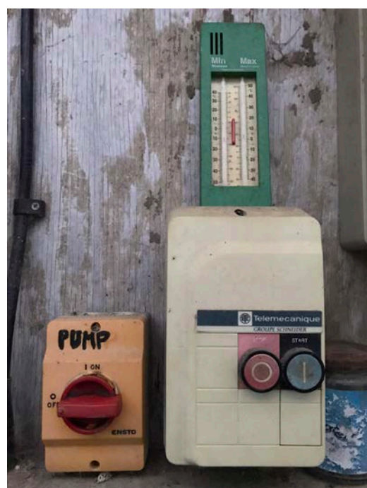
Pump DOL (Direct On-Line) starter and overcurrent device
