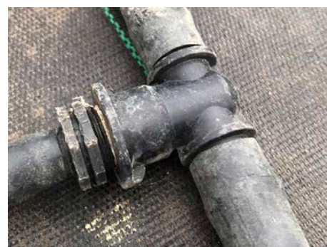
19mm LDPE Manifold to barbed Tee with 1/2" threaded branch to a director for drip line connection
