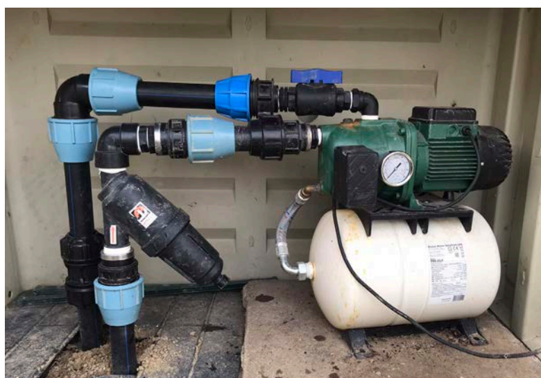
Horizontal pump with expansion vessel , intake filter and automatic pressure switch set-up in a plastic garden storage box. The Montessori Place.
